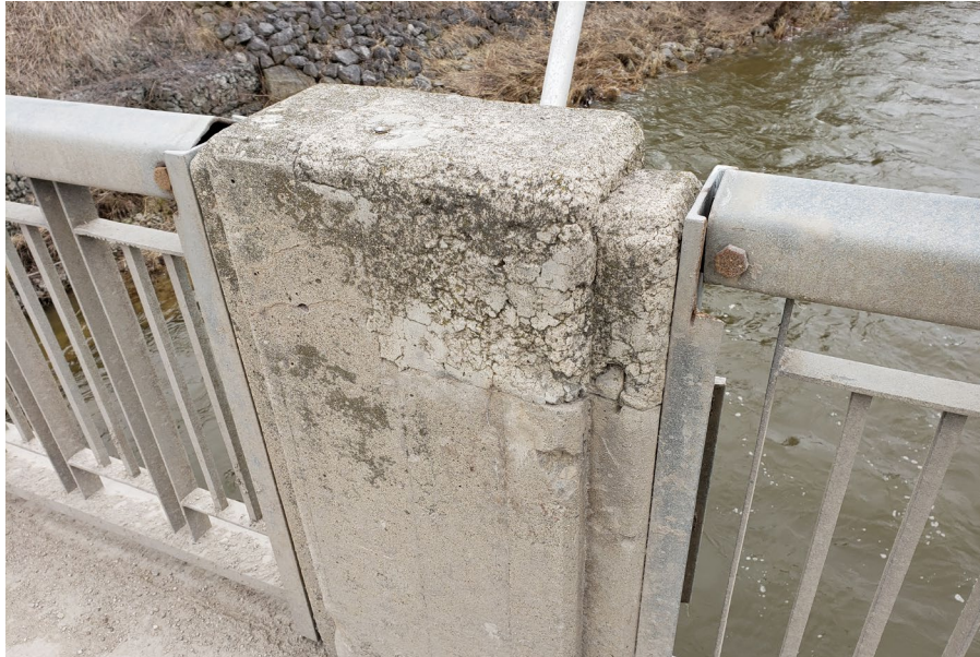
Image 28: Concrete railing post deterioration north side (TMHC 2021)
