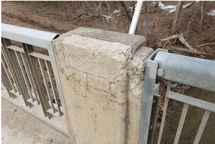
Image 27: Concrete railing post deterioration north side (TMHC 2021)
