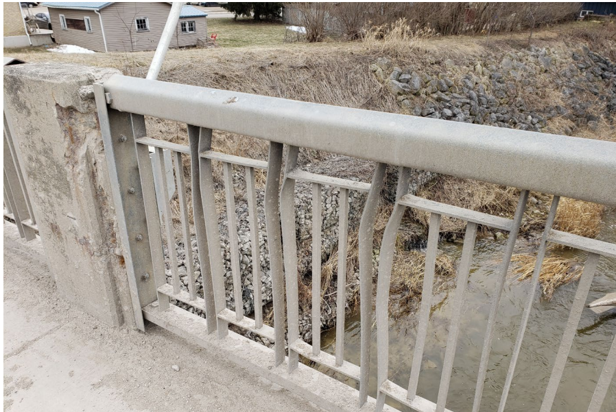
Image 31: Railing damage southeast side (TMHC 2021)
