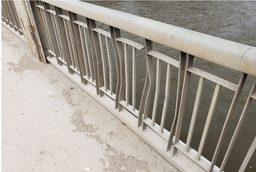
Image 32: Railing damage northeast side (TMHC 2021)
