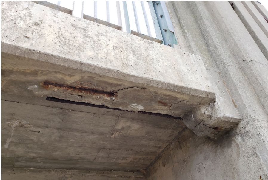
Image 34: Concrete deterioration (TMHC 2021)
