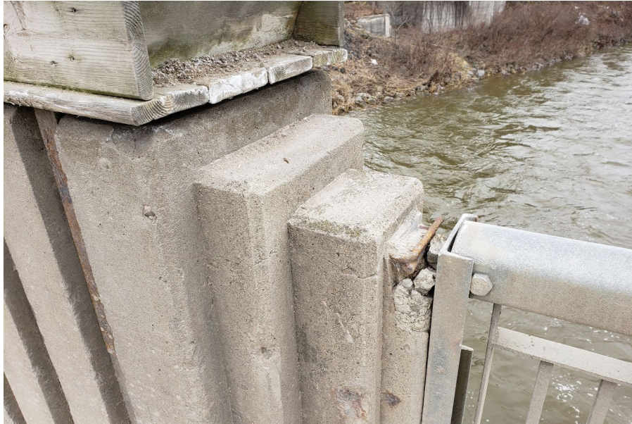
Image 24: Representative image of stanchion deterioration particularly at railing joints (TMHC 2021)
