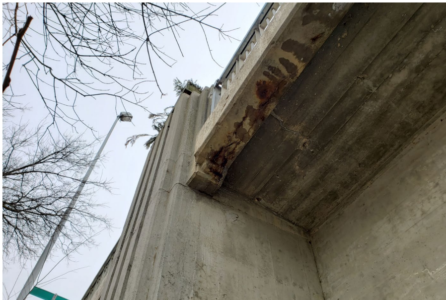
Image 35: Concrete deterioration (TMHC 2021)
