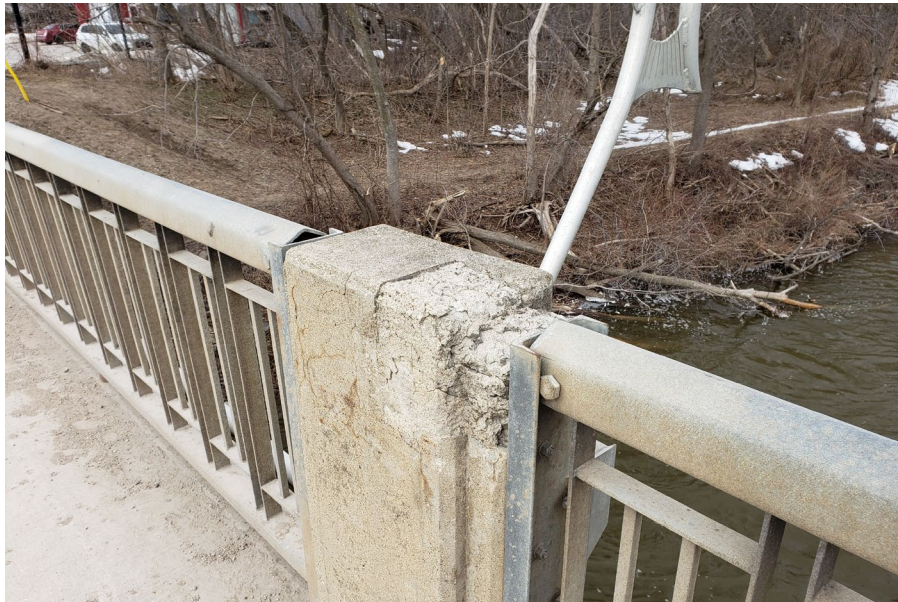
Image 29: Concrete railing post deterioration north side (TMHC 2021)
