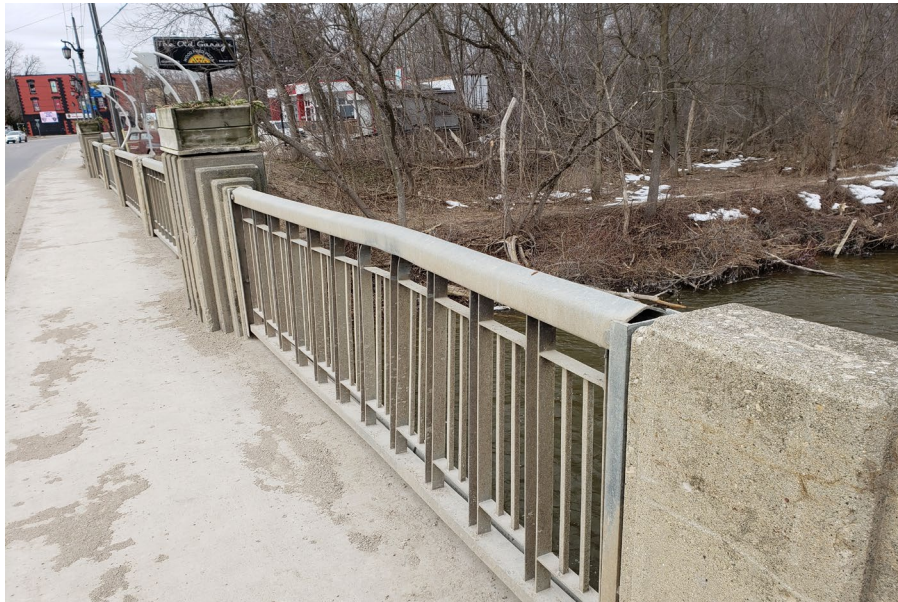
Image 33: Railing impact damage north side (TMHC 2021)
