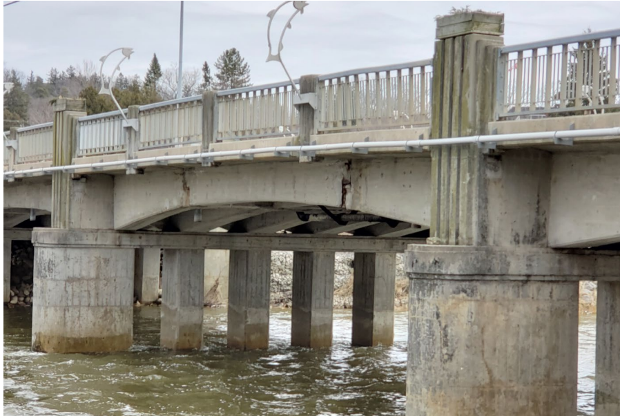
Image 20: Drop-in center span with visible deterioration of half-joints (TMHC 2021)
