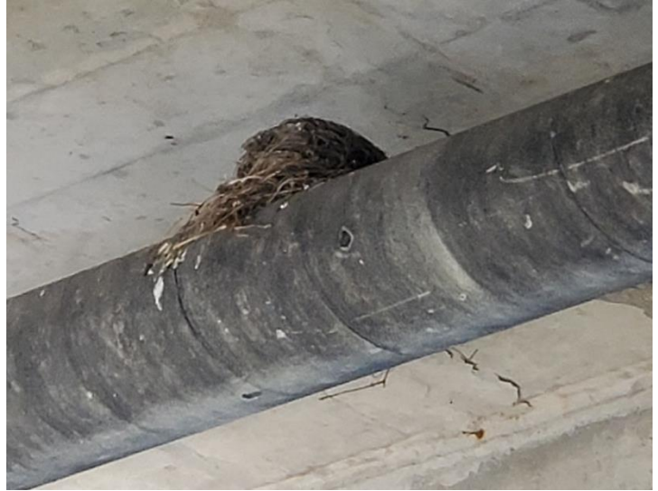
Bird nest observed under bridge ↑
