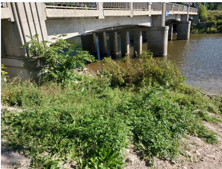
Vegetation on southwest bank of bridge ↑
