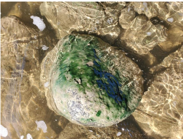
Algae observed on rocks under east side of bridge ↑
